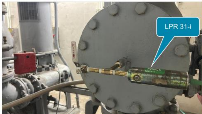
Figure 3.1 LPR 31-i Monitoring Location
