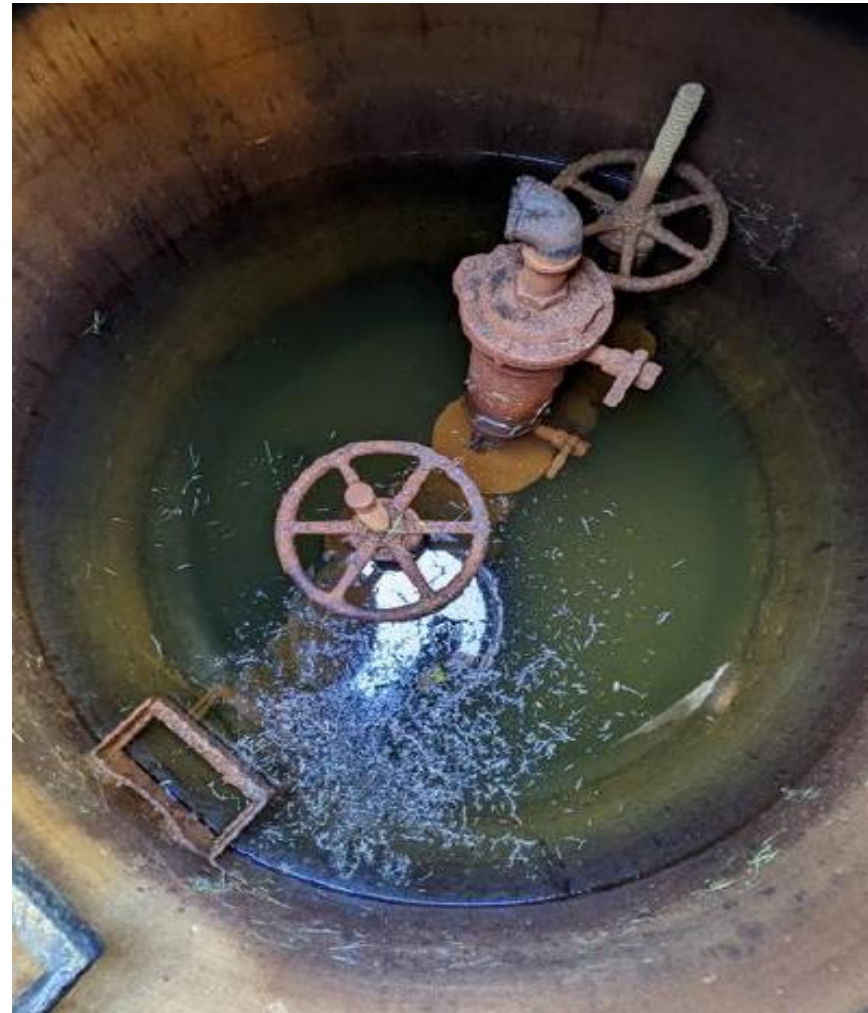
Flow Control, Clean Out, and Air Release Valves
