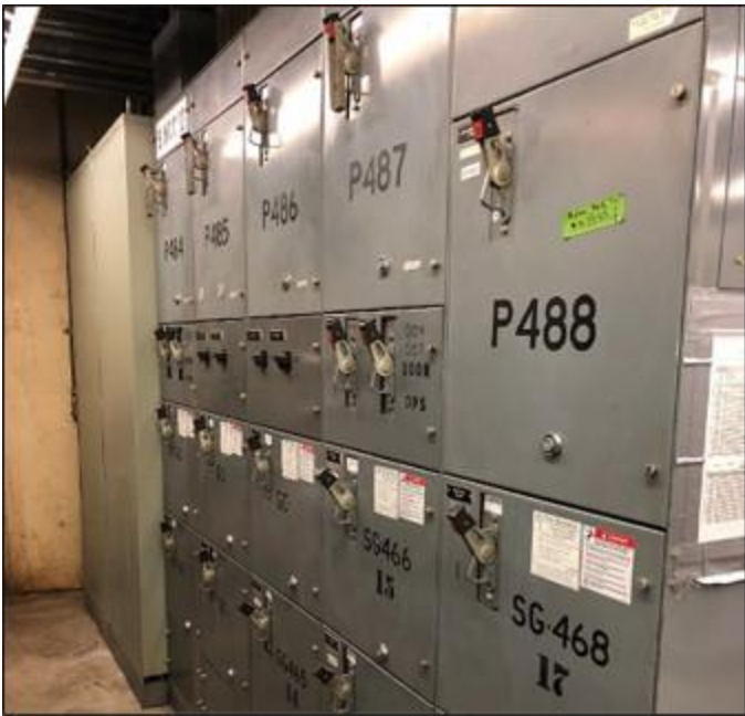
Motor control center
