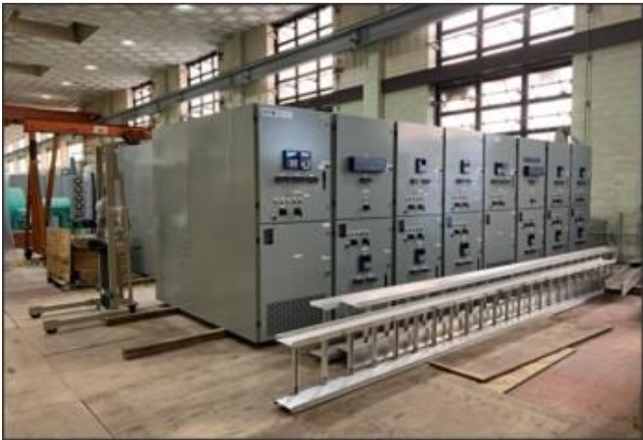
New unit substations to be installed
