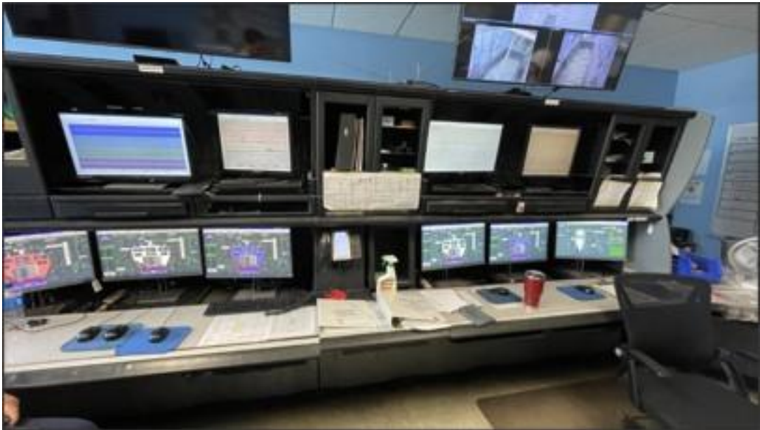
Existing Metro WRRF Solids Management Building Control Room Built in 2004
