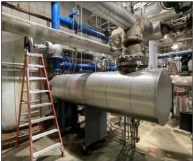
Existing Auxiliary Condenser to be Replaced
