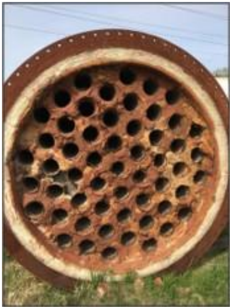
Existing Primary Heat Exchanger to be Rehabilitated
