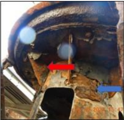
Gravity Thickening Metal Repair
