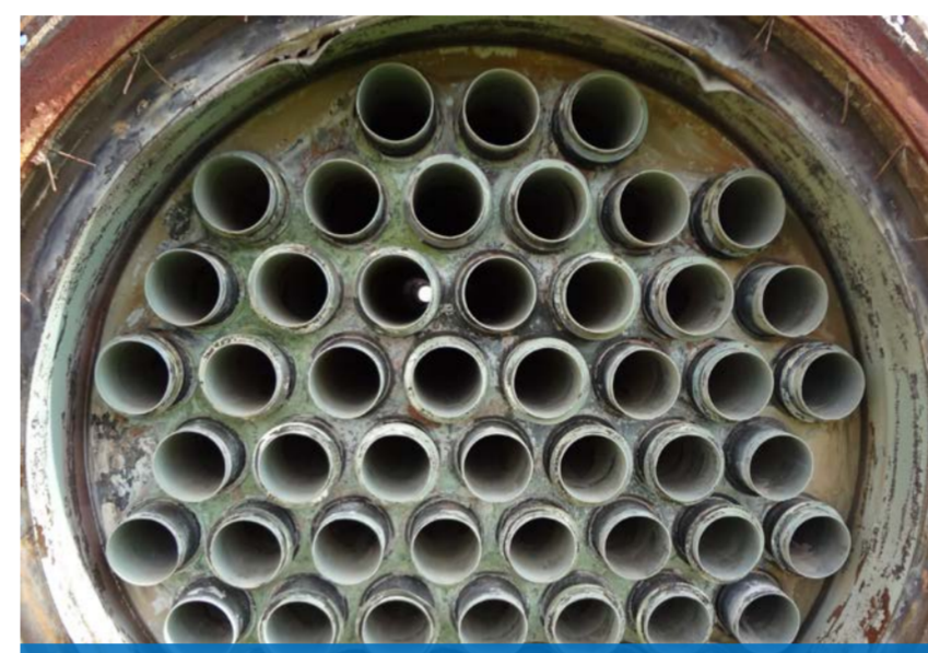
Primary Heat Exchangers
